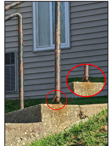
Figure 2 - Rusty, detached hand railing at Tompkins.
