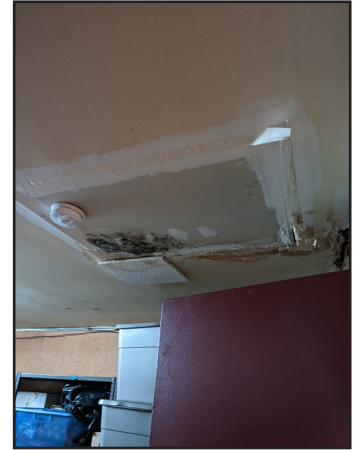
Figure 1 - Water-damaged ceiling in Barker storage room.
