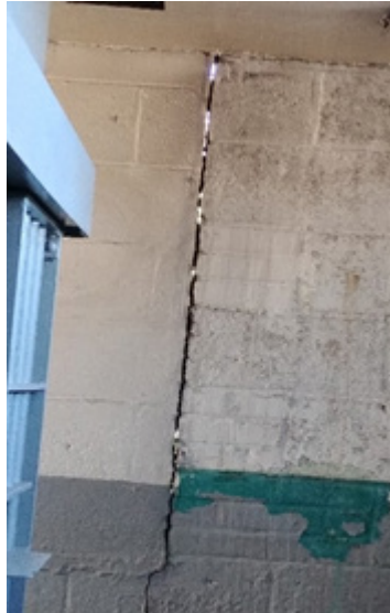
Jail Cell Wall Crack
