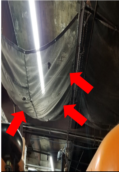
Ceiling Debris in the Highway Garage
