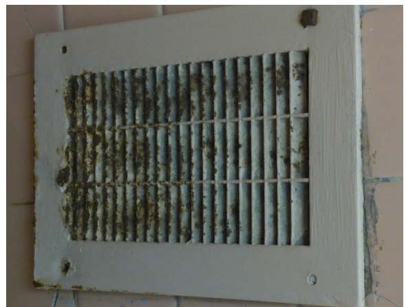
Figure 4 – Dirty, Rusting Air Vent
