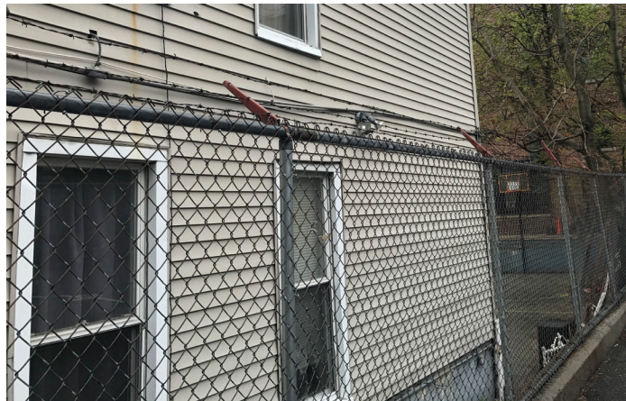
Figure 9 – Barbed Wire on Top of Climbable Chain Link Fence
