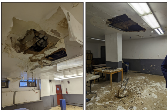
Figure 1 – Partially collapsed ceilings in the Classon community room due to major active water leak.
