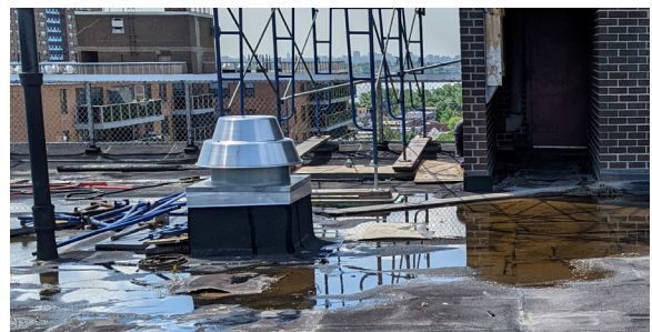
Figure 5 – Jamie Towers, Building 2 roof damage.
