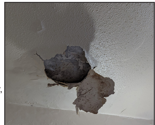
Figure 4 – Unrepaired water-damaged ceiling posing health and safety hazards to the tenant living in the unit.
