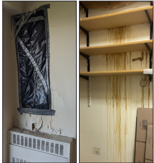
Figure 3 – Water damage in vacant Classon units.
