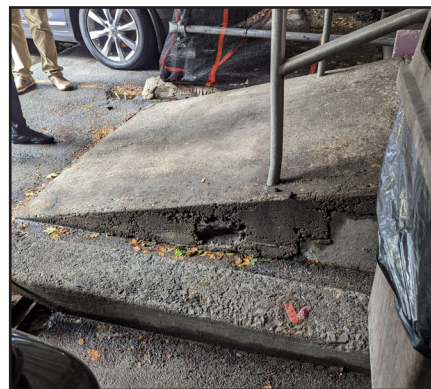
Figure 2 – Steep entrance ramp from Classon parking lot where a resident fell.
